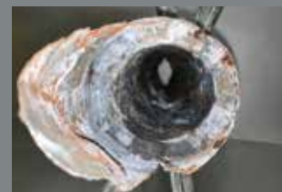
Sludge and initial signs of corrosion on the circuit
