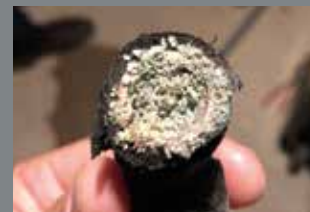
The thermostatic valve Y-strainer clogged on the distribution
