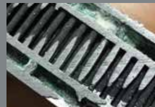
Cross section of a corroded heating unit body
